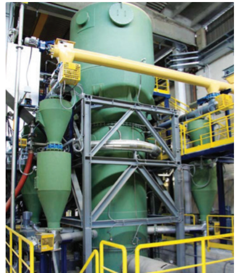
Fluidised bed gasifier using EQTEC gasifier technology
